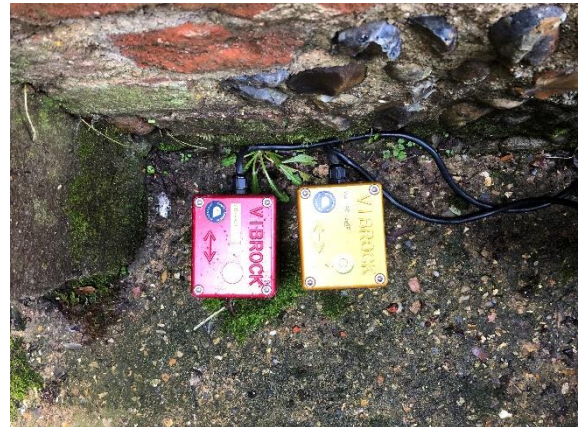
Figure 3.7: Vibration Monitor at 20 High Street
